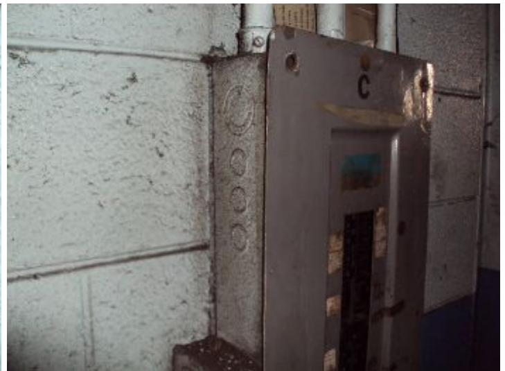
Panel cover screws missing
