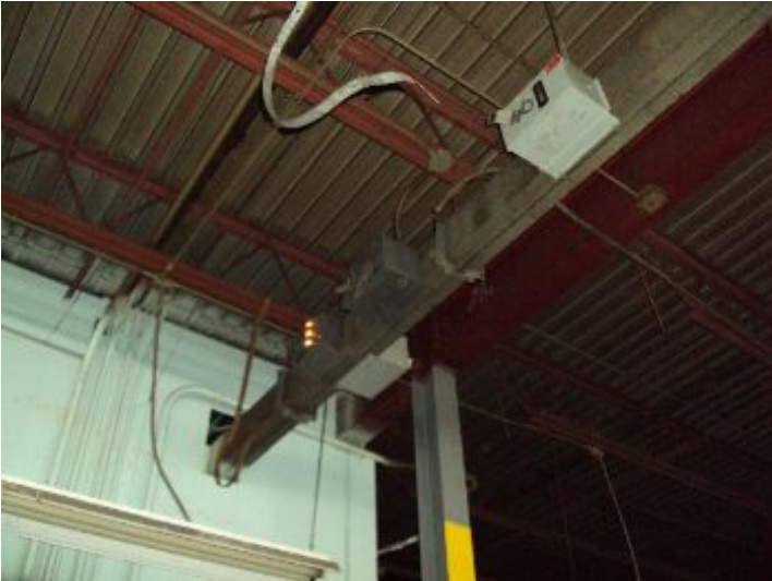
Bus duct with panel disconnects
