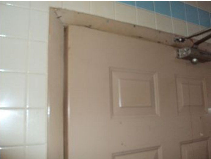
Men's room door does not close properly
