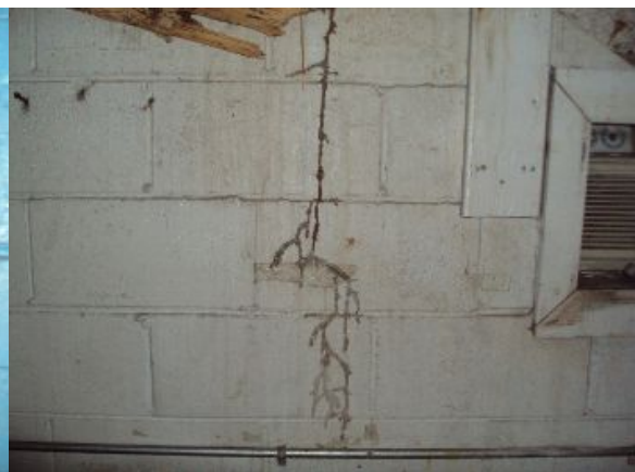
Termite shelter tubes in receiving office.
