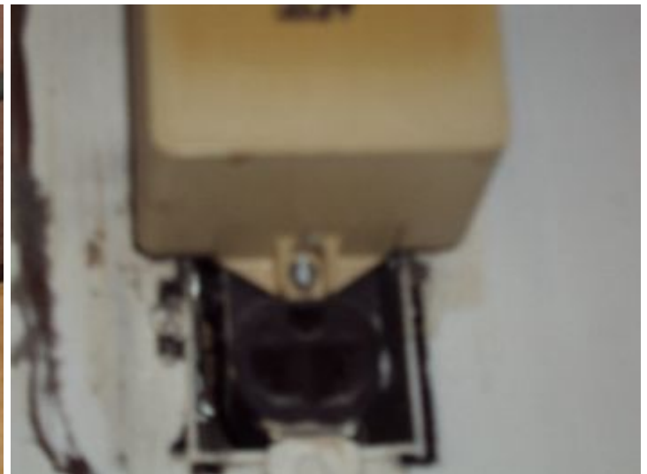
Missing cover in office space
