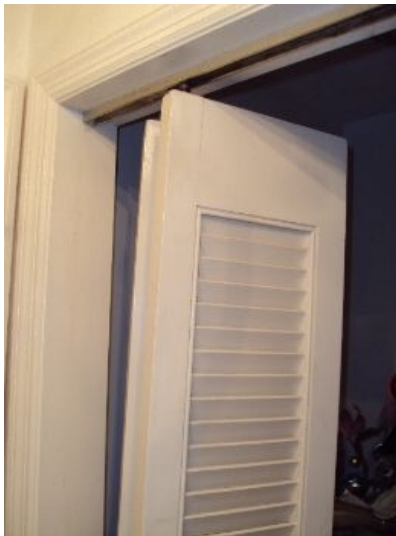
Door out of alignment
