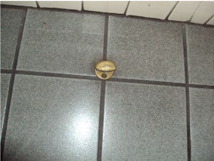
Door stop in womens room crushed and ineffective
