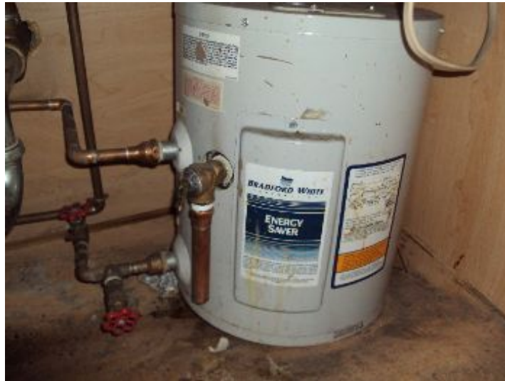
Water heater support damaged.
