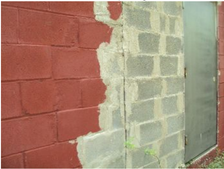
poor quality masonry
