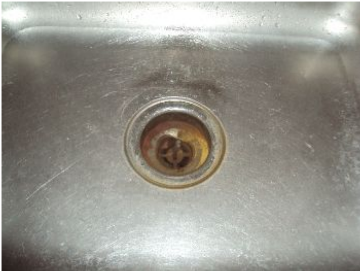
Sink drains poorly.
