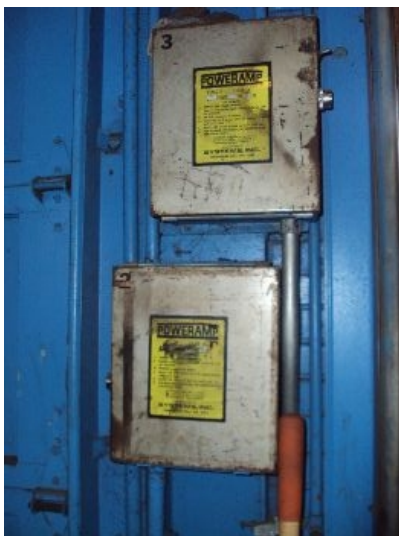
Dock leveler controls
