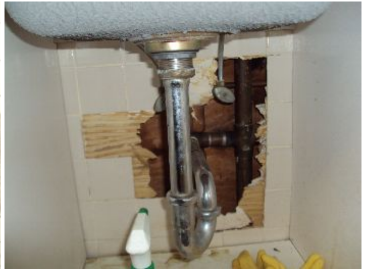
Evidence of a prior repair (Mens Locker Room)
