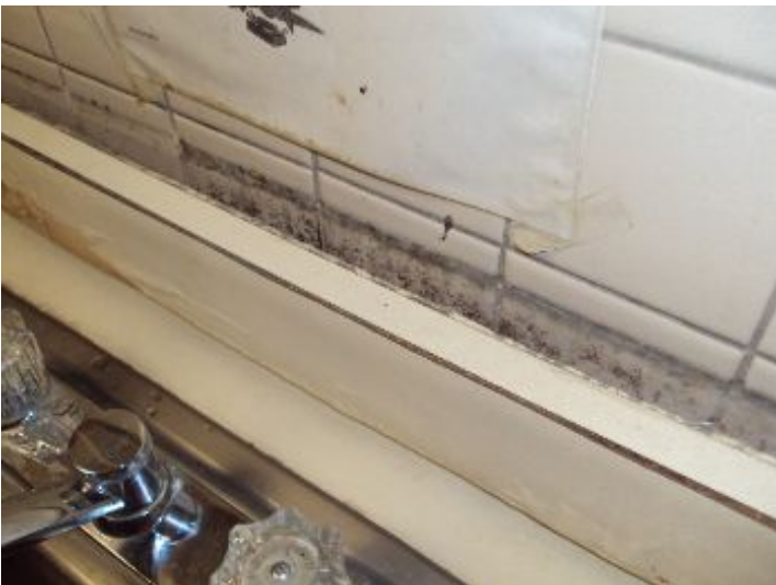
Backsplash water damaged and coming loose
