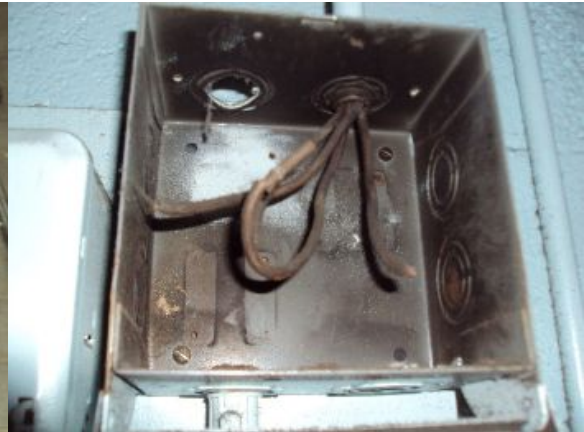
Abandoned electric in closed box
