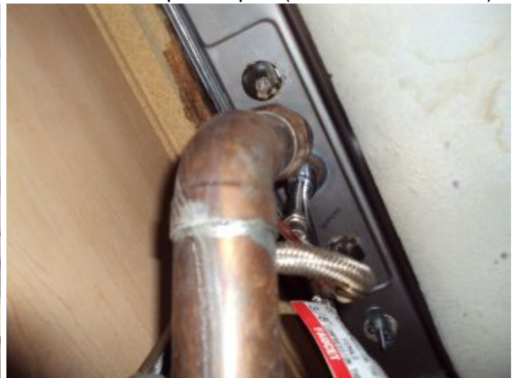
Air admittance vent. No AAV installed.
