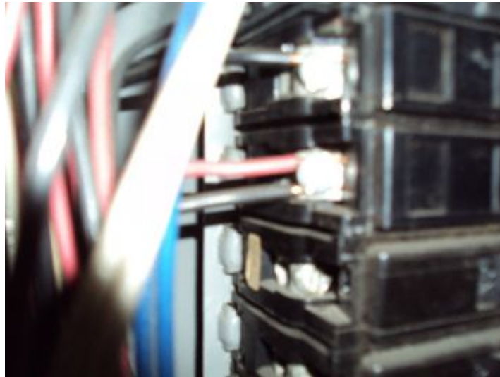
Double tapped breaker noted.
