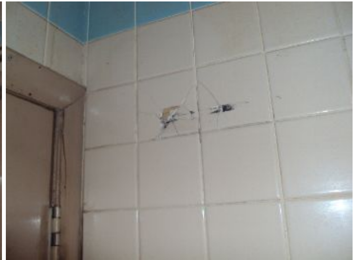
Damage to ceramic tile from door closer arm
