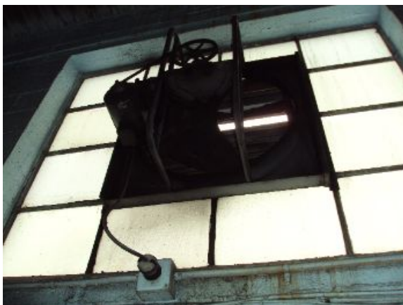
Exhaust fans not tested
