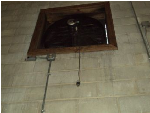
Ventilation fans not tested
